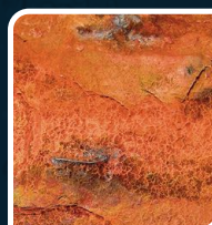
Corrosion and rust
